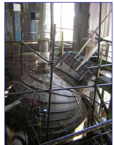
Upper surface of a urea stripper in Iran
