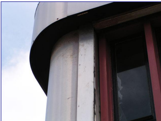
Staining on stainless steel facades
