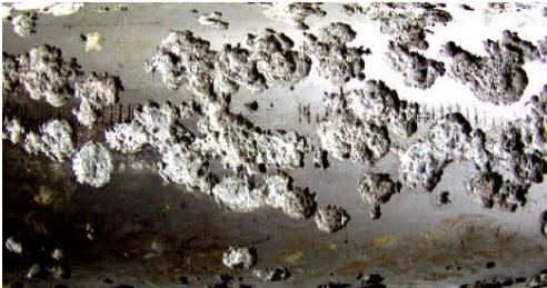
Pit corrosion to AISI 316 pipe
