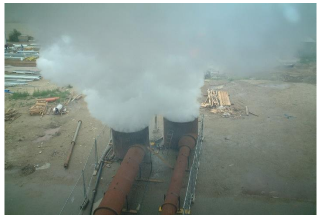
Steam separator (condenser)
