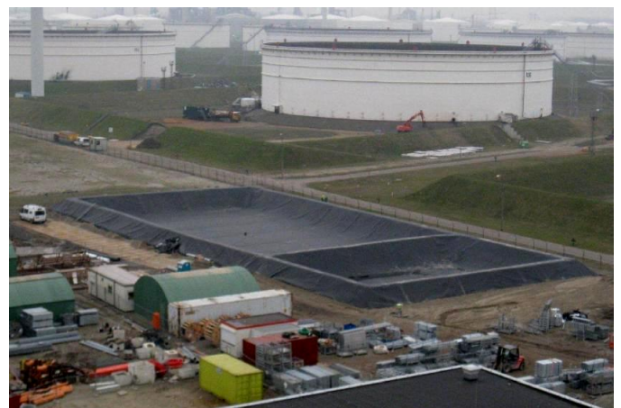
An effluent pit after the earthworks (top) and the final result (bottom)
