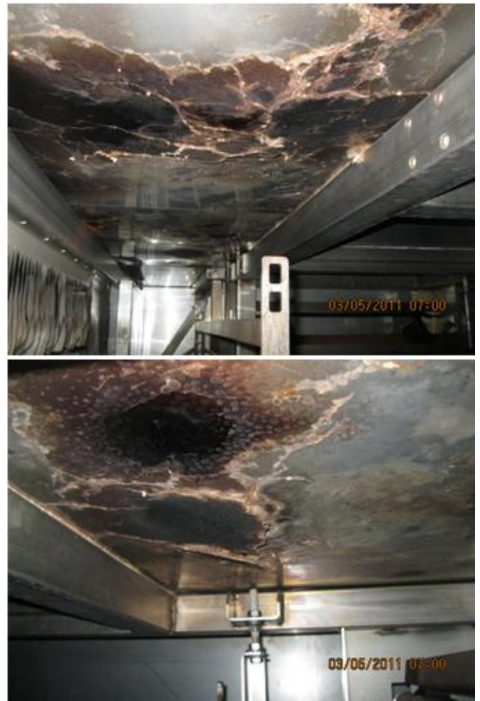
Intergranular corrosion in an oven (Photo: Cobra Consultancy)
