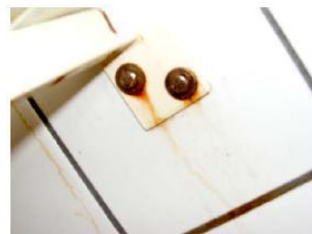
Heavily corroding stainless steel parts
