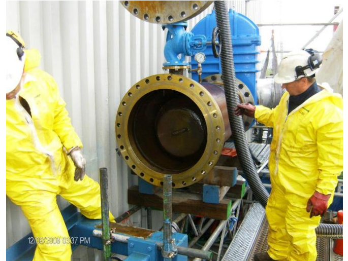
Fig. 2: Pipe pigging launcher
