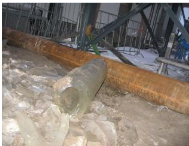
Photo 4: ice removed from demin-water line
