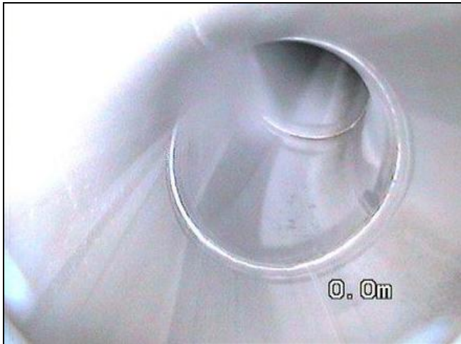
Photos and boroscope inspection of line 5SB – successful pickling
