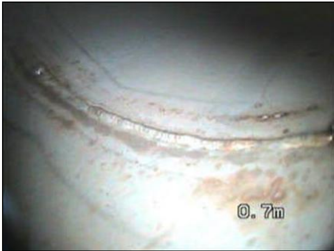
Line 5SB (before treatment) – Weld seams contaminated with significant corrosion products
