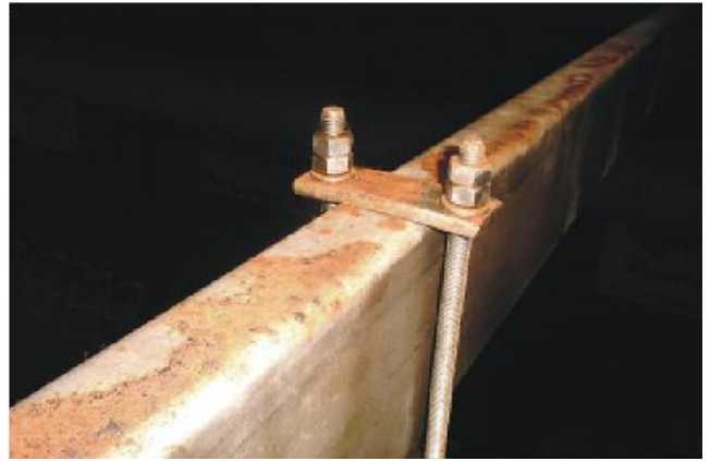
Serious form of corrosion in supporting stainless steel constructions.
