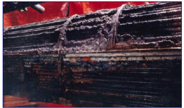
Figure 2: Contamination of a heat exchanger with the cooling water on the shell side
