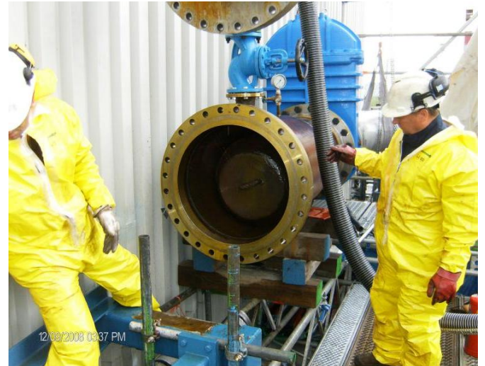
Afb. 2: Pipe pigging launcher
