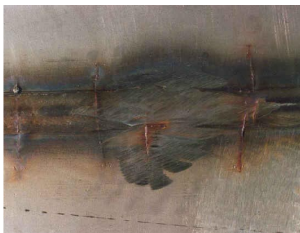
Foto 1 Scheurvorming in X2CrNiMoN22-5-3 MVC strippers
