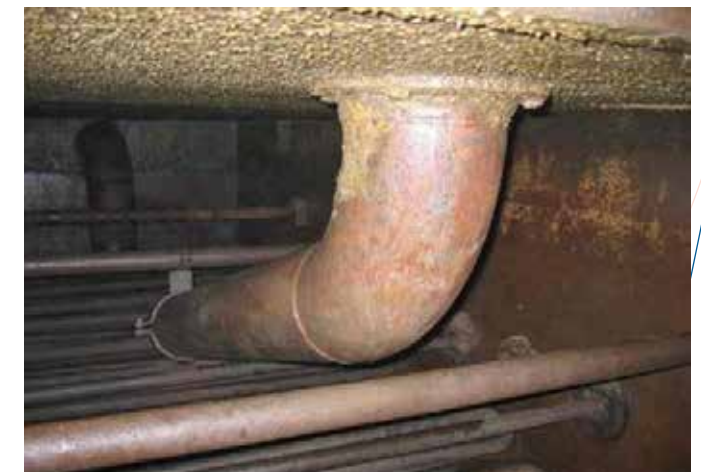
Smeerolie tank (25 m 3 ) na reinigen
